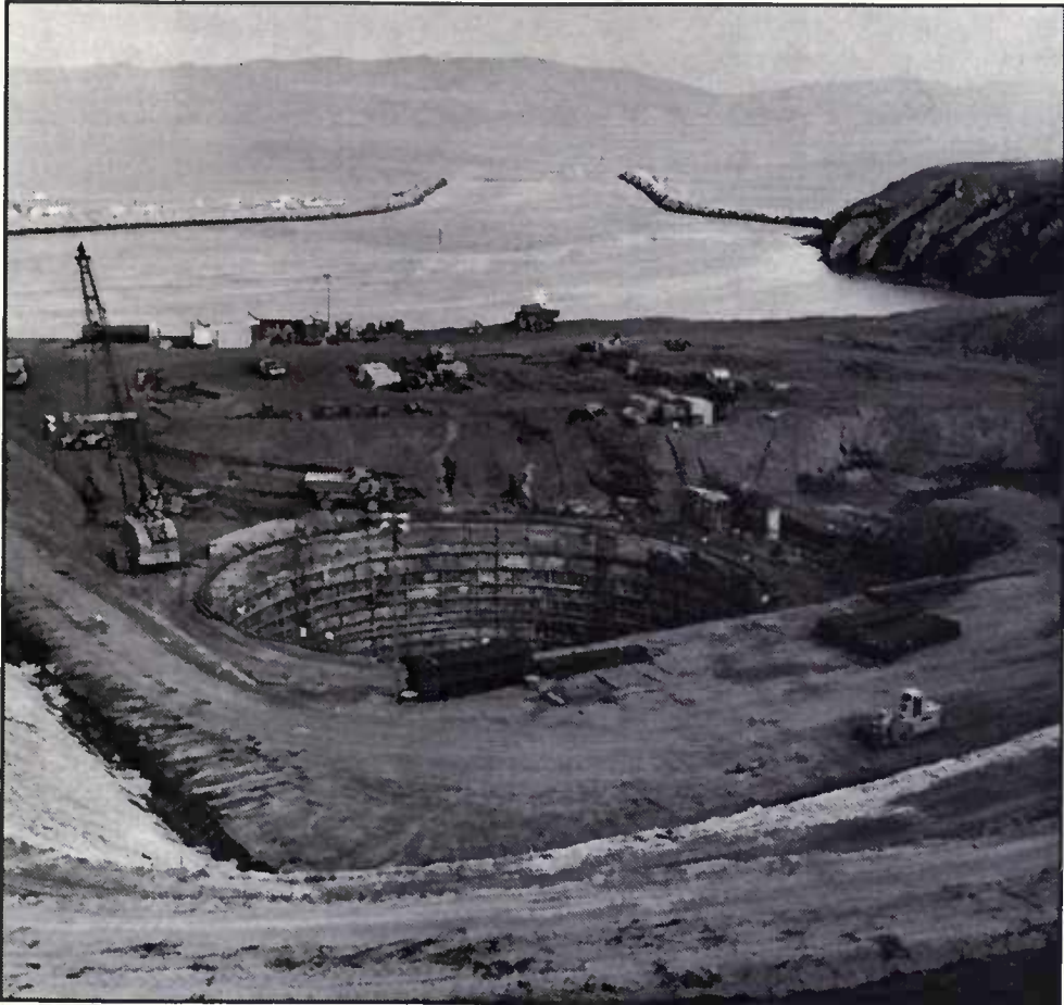
The Hole in the Head, nuclear reactor under construction at Campbell Cove, Bodega Bay.
