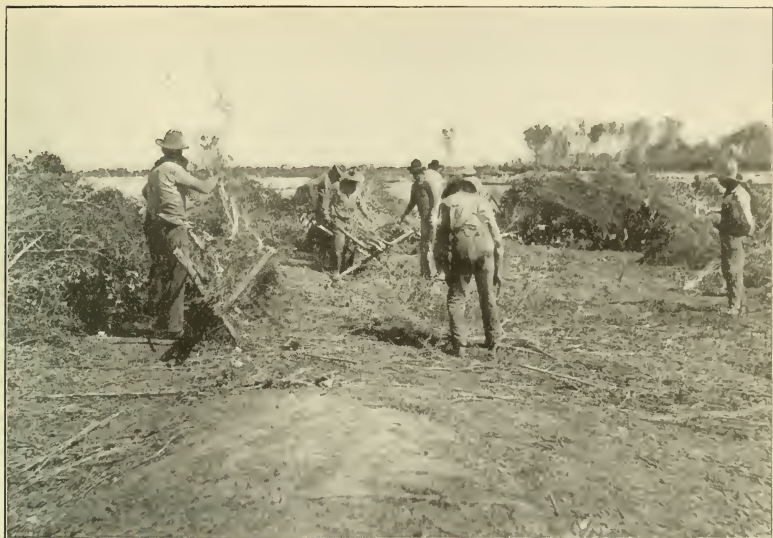
Preparing Brush for the California Development Company's Dam in the Colorado River, Just Below the Old Bed of the River.
